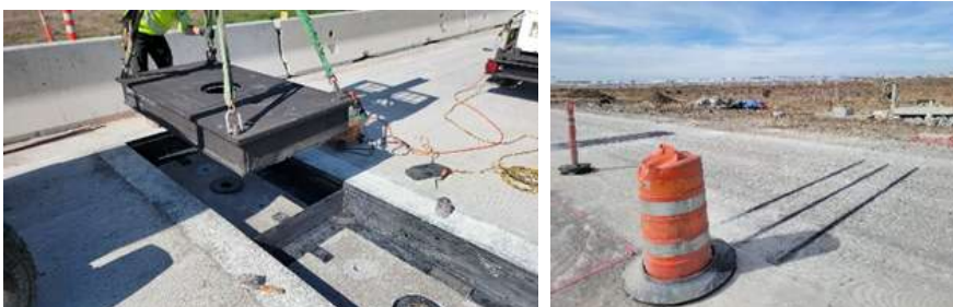
SLC WIM Scale and TACS Installation – Declo Idaho
