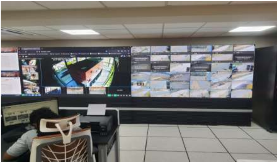
The Data Center at the KeNHA headquarters
