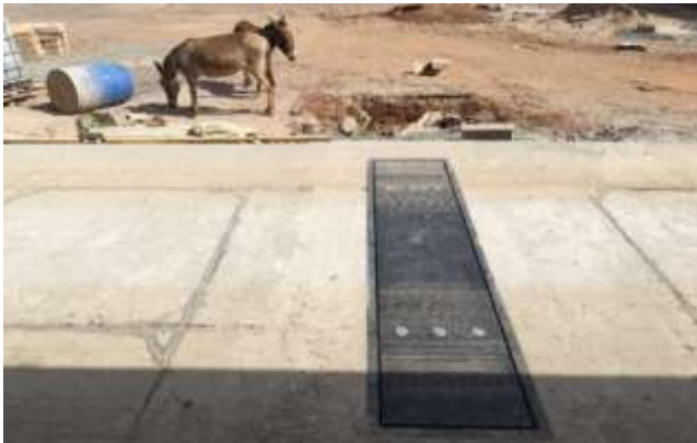
An 4020 low-speed WIM Scale installed at the Sotracom Aggregate Facility
