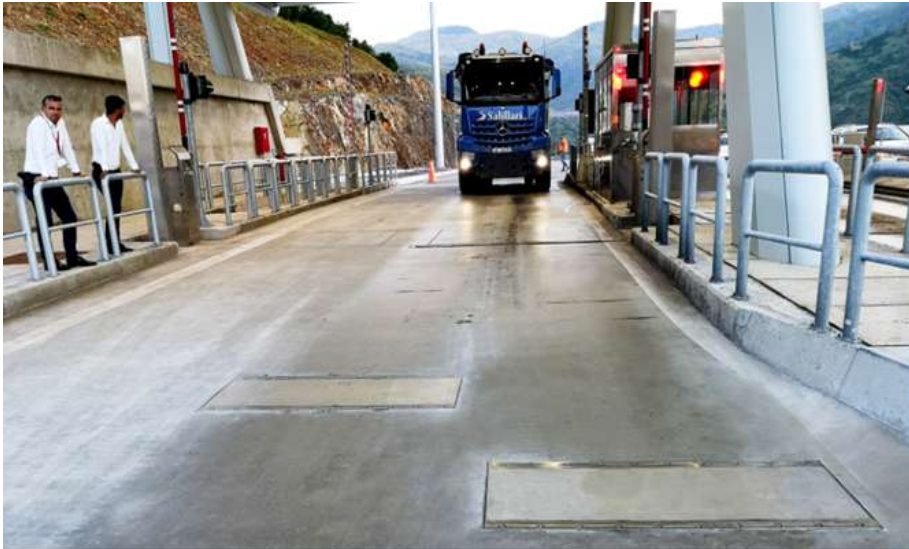
BISON installation on the Kukës motorway toll gate
