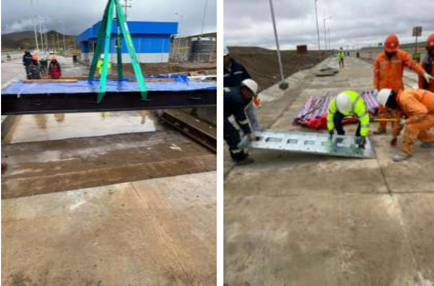
Installation of GirWIM LS and MS WIM scales in South America
