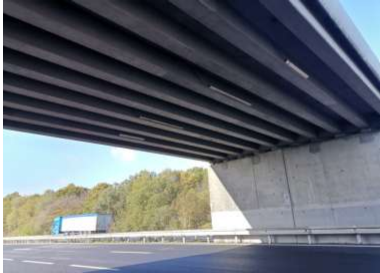
WIM+D system under the Auzouer bridge in France.
