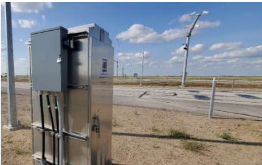
Virtual Weigh Station Site on the Regina Bypass
