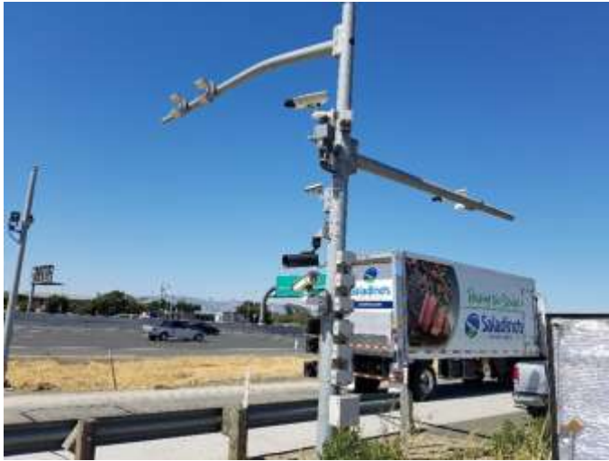
Ramp Screening Technology – Cordelia, CA
